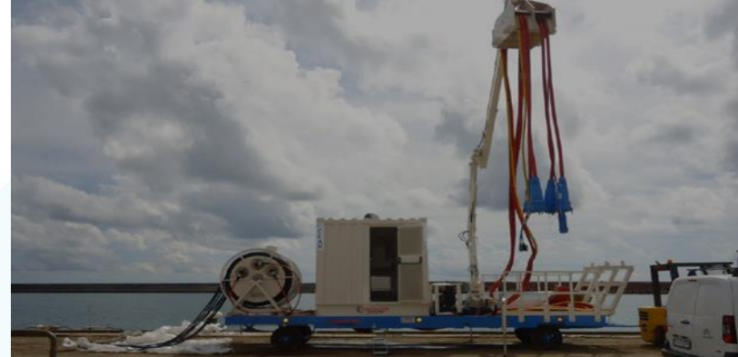
Figure 3: Port of Genoa – Onshore Power Supply
